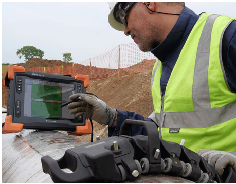
Figure 1: Operator performing in-field data analysis during a pipeline inspection using a Spyné™ ECA probe, Reddy® instrument, and Magnifi GO software.
